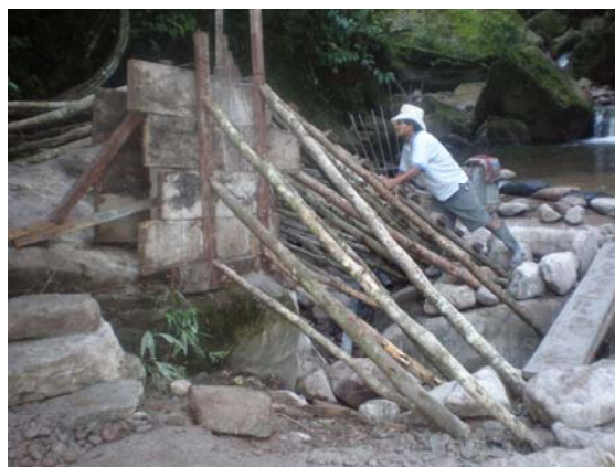
Figure 3: Civil engineering for a micro hydro scheme in Bocatoma, Peru. Photo: Soluciones Prácticas.
